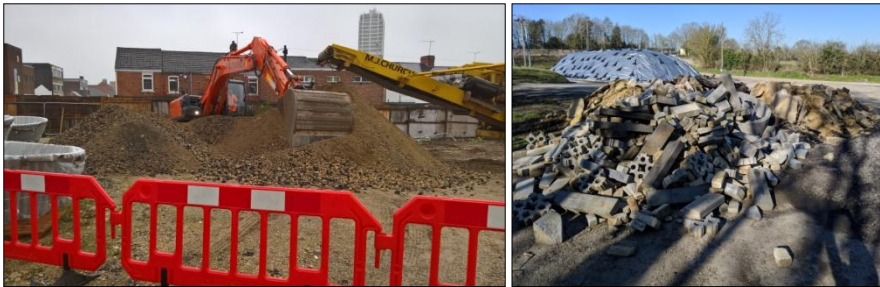
Waste concrete is being crushed for reuse in verge and other repairs
