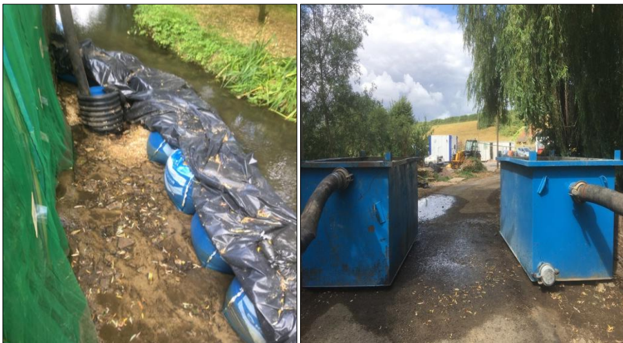
Filtration tanks can be used as part of the over pumping operation
