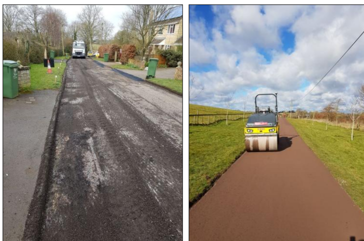
In-situ recycling makes use of the existing road material by excavating and mixing it and treating it to increase its strength
